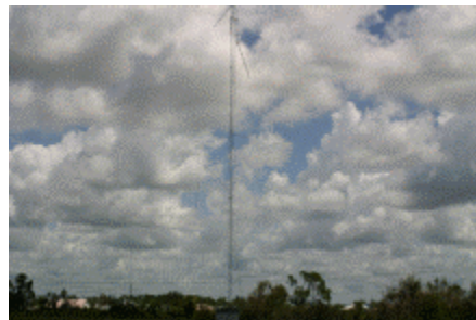
This was a Rohn 25 tower. The top 30 feet is bent to the right, and the hardline is all tangled in the guys.
