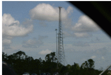
7/8-inch hardline literally ripped off the side of this cell tower. Even the ladder bolted to the tower was ripped off.
